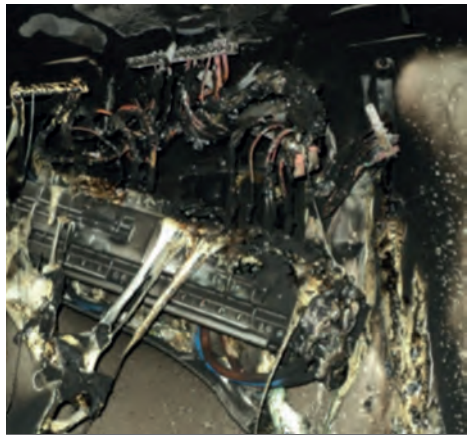
Fig 1. Consumer unit with plastic enclosure after a fire caused by a loose neutral termination
